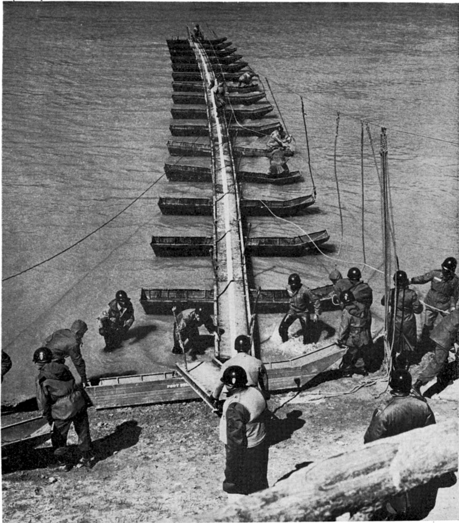
THEY PAVE THE WAY . . . Members of the 72nd Engineer (Combat) Company, Second Battle Group, 14th Infantry, pave the way for a river crossing by constructing a foot bridge for the oncoming troops.
