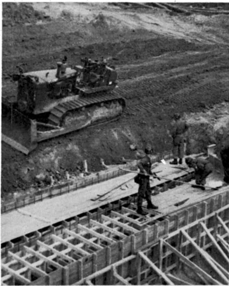
MEMBERS OF COMPANY C, 806TH BATTALION Prepare Form Work for Concrete Box Culvert
