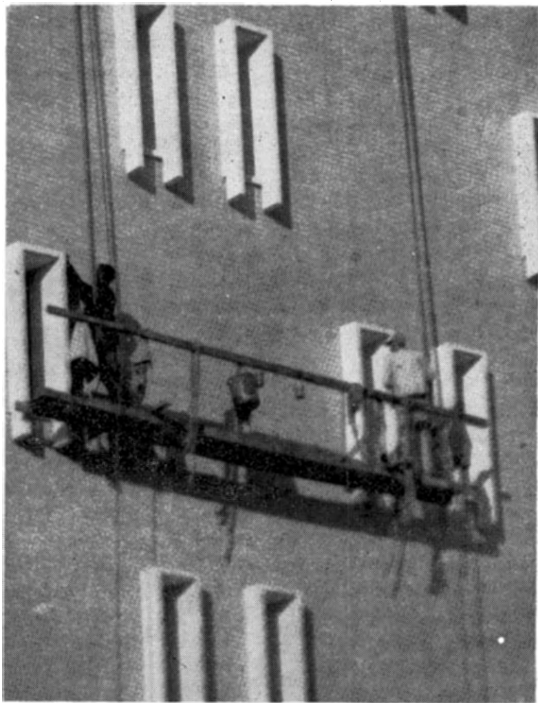
Some of the finishing touches are put on the face of the new Infantry School Academic Building, one of the projects of Infantry Center and Savannah District Engineers. Chief of the post Engineer Division, Simeon Cox, says, "We are way ahead of schedule on the Academic Building. It would not be sticking our necks out too far to picture its completion before May."
